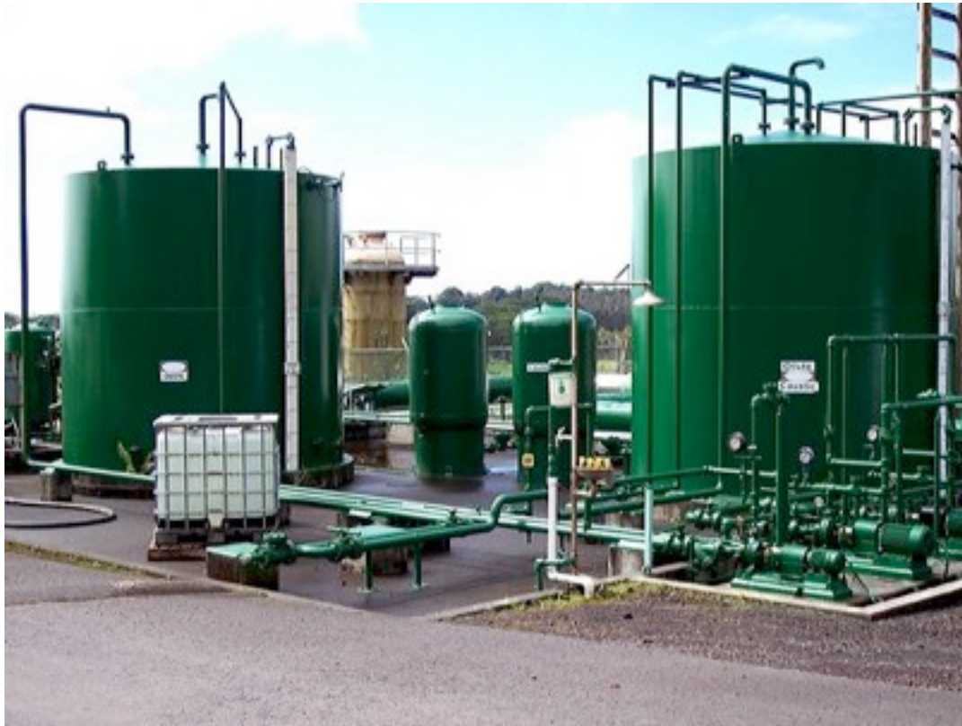
Puna Geothermal Venture facilities
