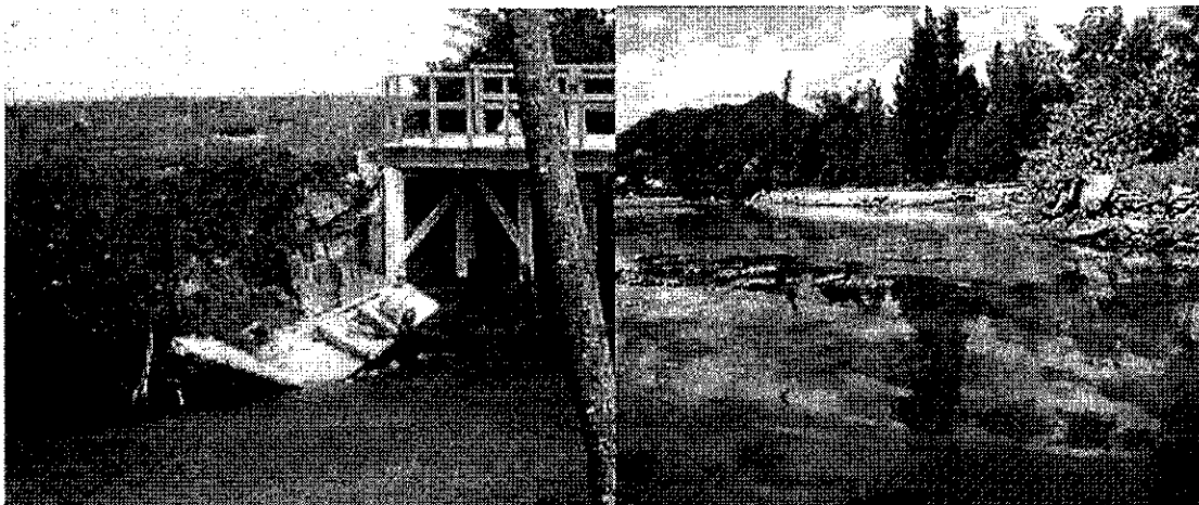
Fallen seawall, inner lagoon
