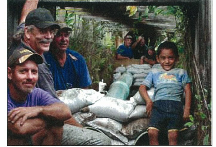
The volunteer crew who fixed it until permanent repairs could be made
