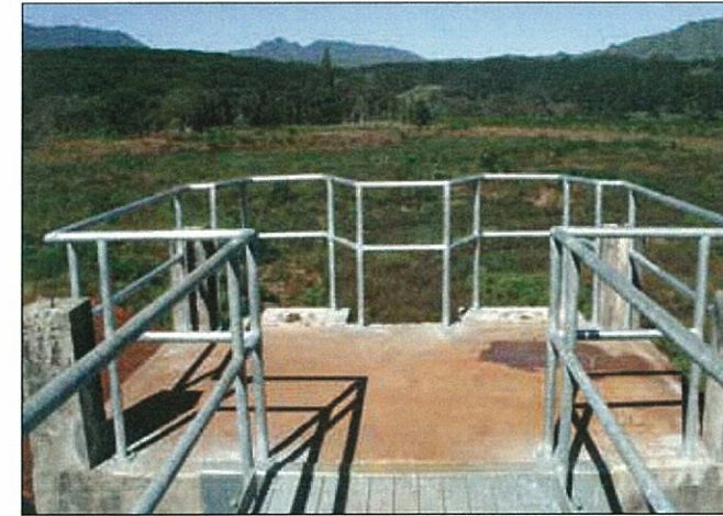
New catwalk and control gates overlooking a drained Wailua Reservoir under repair
