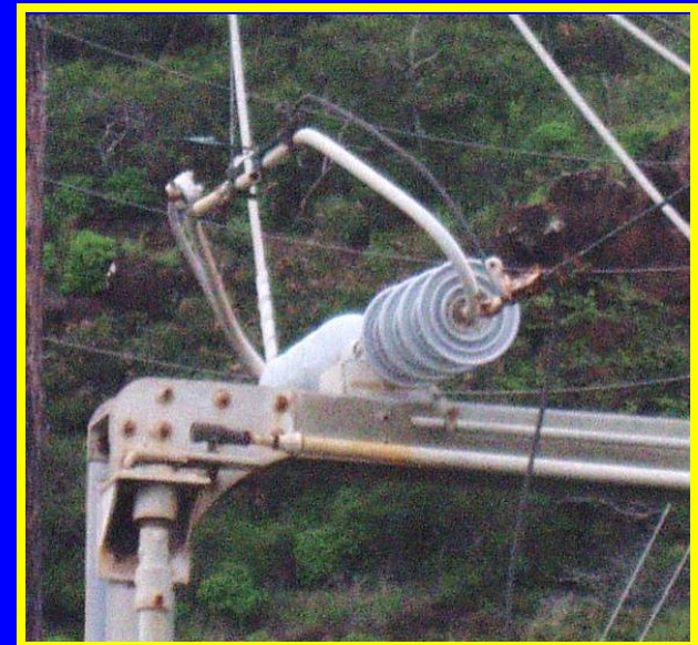
Closed Switch 46kV
