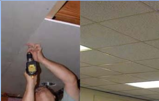
Ceiling Fixed Gypsum board Acoustical Tile Grid
