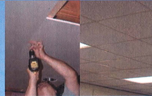
Ceiling Fixed Gypsum board Acoustical Tile Grid
