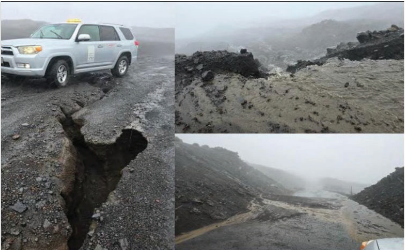
Figure 9. Hurricane Hone Damage.
