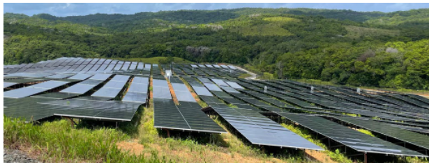
Figure 1. PV arrays at Palau's SPEC PV+BESS plant.
