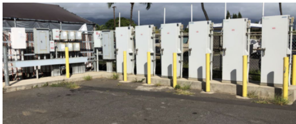
Figure 1. Sunverge SIS BESS + PV units on Maui.
