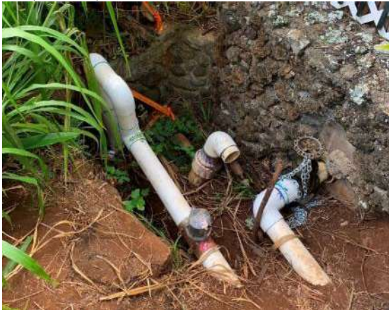
A) Distribution pipe with valve chained and flow meter at center, located on the boundary of Imua Family Services property.
