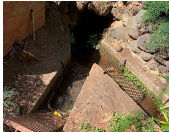
D) Water flows from a driveway culvert at the Velez property and towards Velez, Ciotti, and Ibara.
