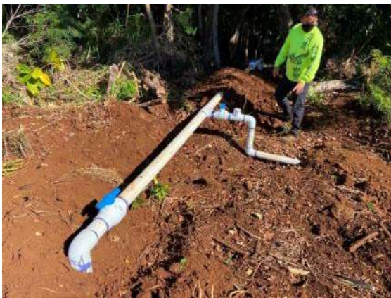
C) Newly installed lateral 4-inch line from Waikapū Properties’ line continues to South Waikapū Kuleana ‘Auwai.
