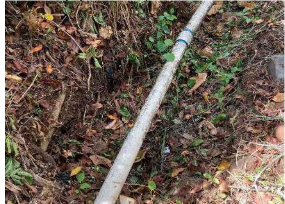
B) An old section of a County water line sits in the ‘auwai, where the water stops flowing approximately 900 feet before the first kuleana user.
