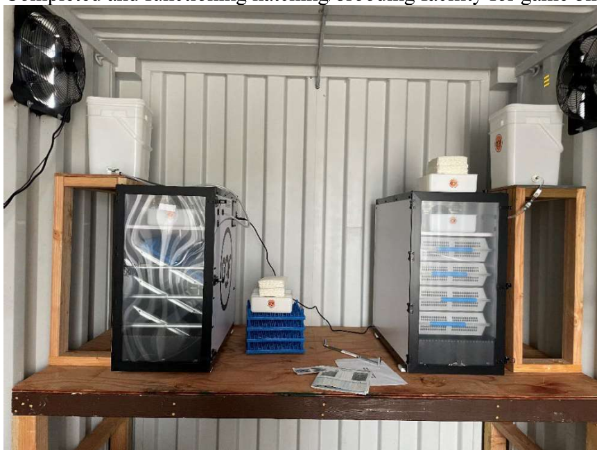
Photo 3. Cabinet incubator and hatcher in the EH Wildlife programs hatching/brooding facility. Electrical and ventilation were installed during FY24 using WLRF.
