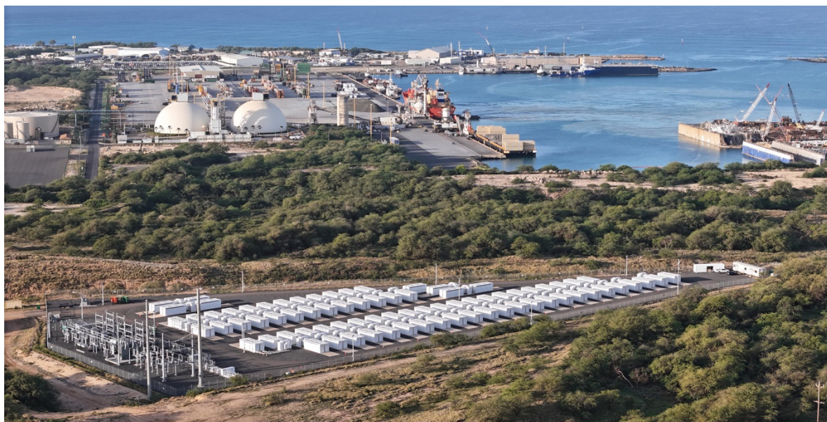
Figure 7 Plus Power Kapolei Energy Storage site. Image courtesy of Plus Power.
