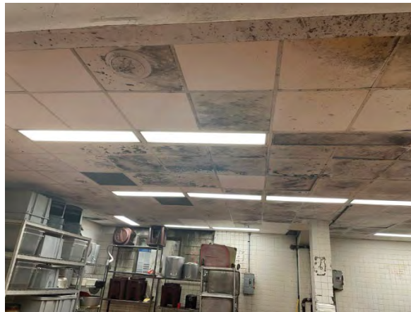
Kitchen Ceiling Tiles
