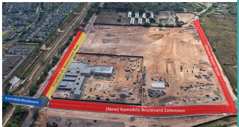
Legend: Closed (Red), Drive with Caution (Yellow), Street Indicator (Blue). The Image Group courtesy of Goodfellow Bros.
