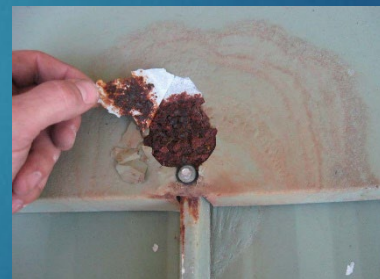
Corrosion of underlying ferrous metal.
