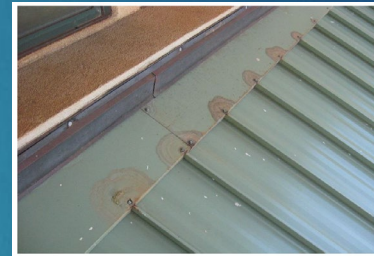
Moderate to severe corrosion of flashing.
