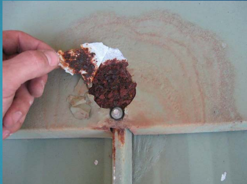
Blistering coating, corrosion of underlying ferrous metal
